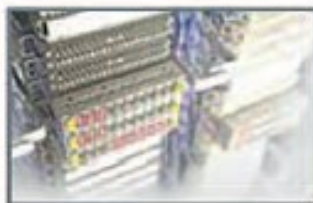
Telecom e ICT2
